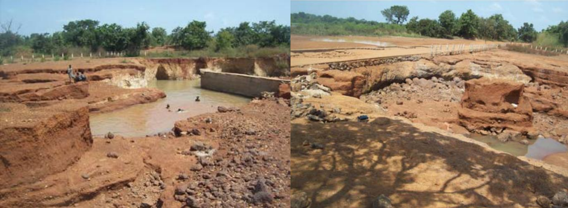
Figure 3 : lateral spillway eroded (source: PNE Benin, 2008)
